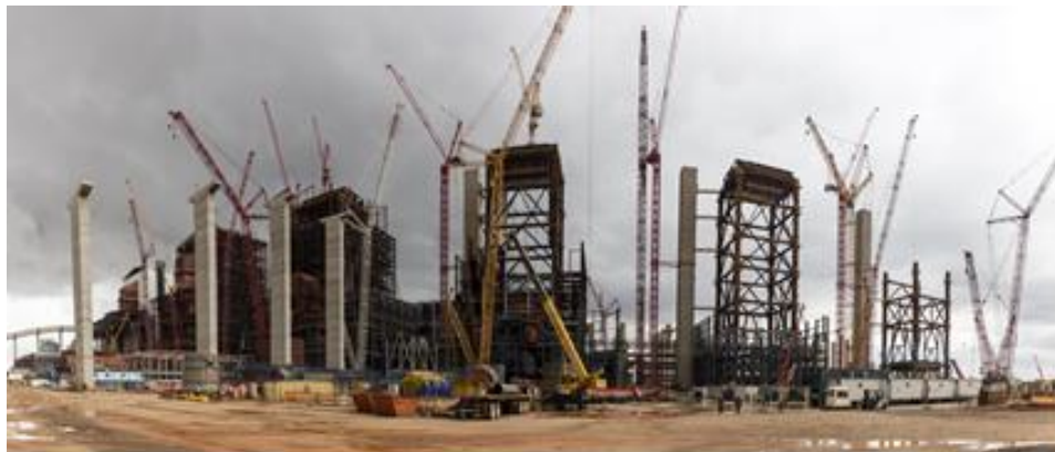
Four WOLFF 1250 B and three WOLFF 355 B are in operation at the Kusile Power Plant construction site amidst a multitude of crawler and lattice boom cranes.
